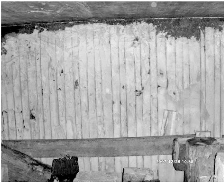
(a) 受损通道盖板钢筋暴露
