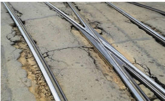
(a) Serious damage of tram track
