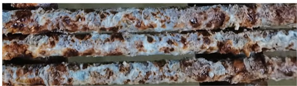
(b) Corrosion time 720 h
