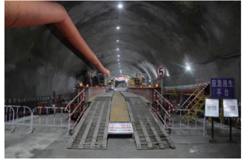
图12 掌子面附近栈桥区段 Fig. 12 Stack bridge segment near the tunnel face
